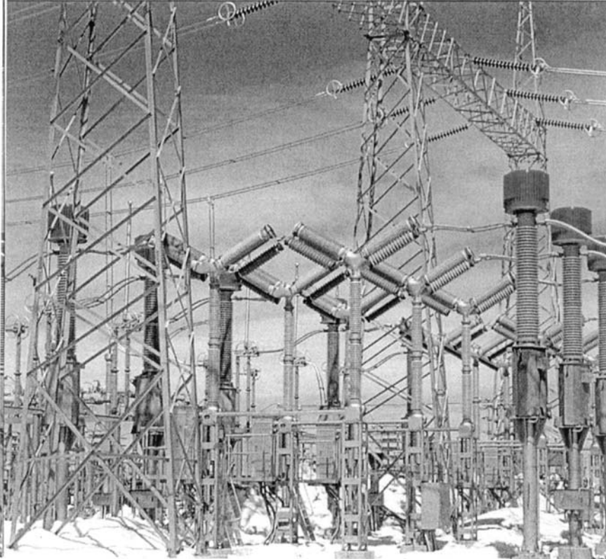
Fig. 6.70 AC breakers and current transformers at Radisson converter station, James Bay, Canada. Design temperature is -50^{\circ}\text{C} . (Courtesy of ABB, Sweden.)
