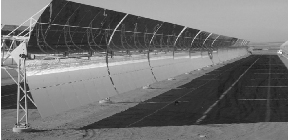
Figure 2.16 50MW parabolic trough plant with thermal storage at Andasol, Spain. (Reproduced from Concentrating Solar Power – from research to implementation. © European Communities, 2007)
