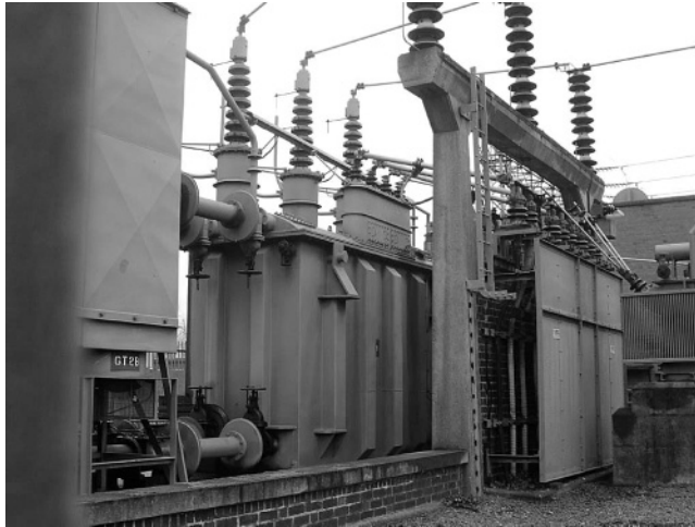
Figure 5.2 Transformer: 132 to 33 kV. (Courtesy of Murray Thomson)
