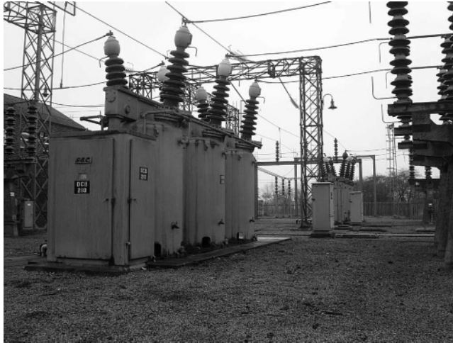
Figure 5.13 A 132 kV circuit breaker. This large and expensive device serves the transformer shown earlier in Figure 5.2. (Courtesy of Murray Thomson)
